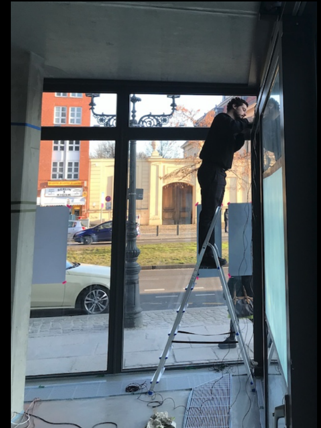
Electrodynamic exciters hidden in the ventilation system and around the architecture of the building
